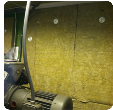
MACHINE ROOM SOUND ABSORPTION
